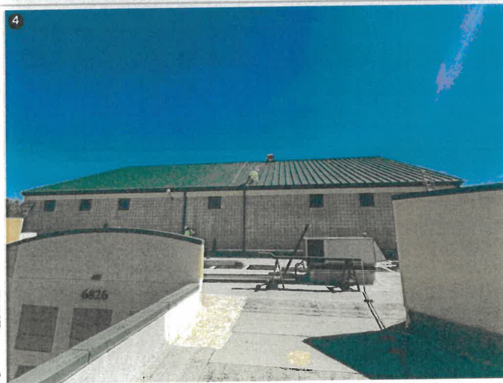
Up close on the flat roof. You can see the crew is building the downspouts and running the seamer. The mechanical seamer is a machine that presses the seam cap together with force.
