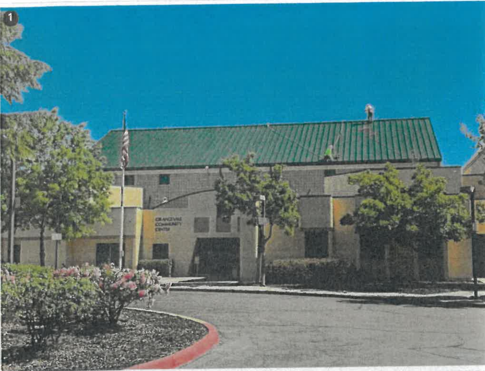
1 Crew is installing the downspouts, running the seamer on the panels and finishing up the roof!
