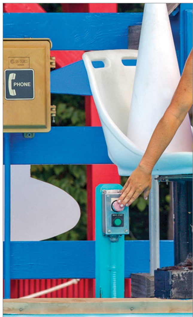
Figure 4-14 | An emergency stop (E-stop) button can be pressed to turn off the waves in a wave pool when a rescue is required.
