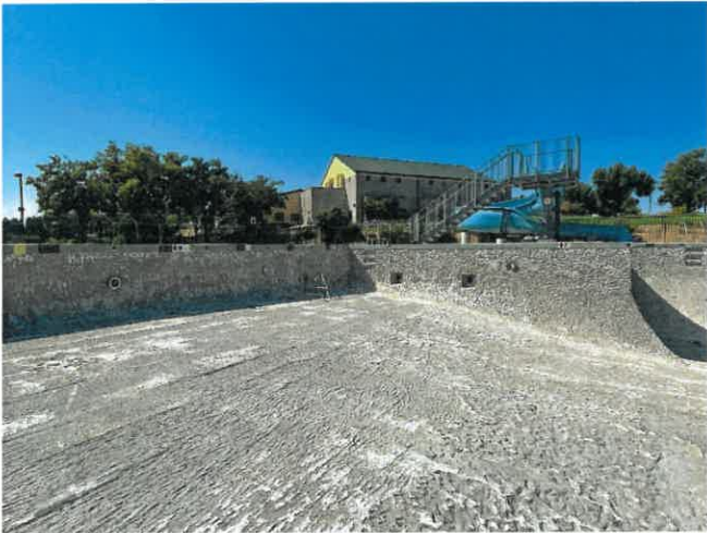
9/23/23 All Plaster is Removed
